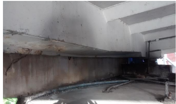
Figure 2: Photograph showing the enclosure in which the bridge bearing survey was carried out using the DiddyBorg robotic platform.
