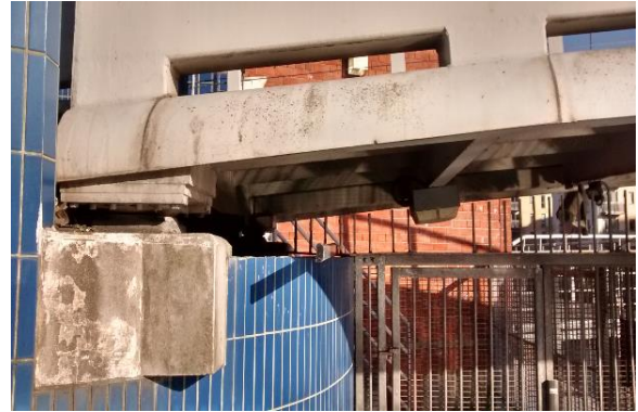
Figure 1: Photograph showing the location of the north-side bearings of Centenary Bridge, Leeds, UK.
